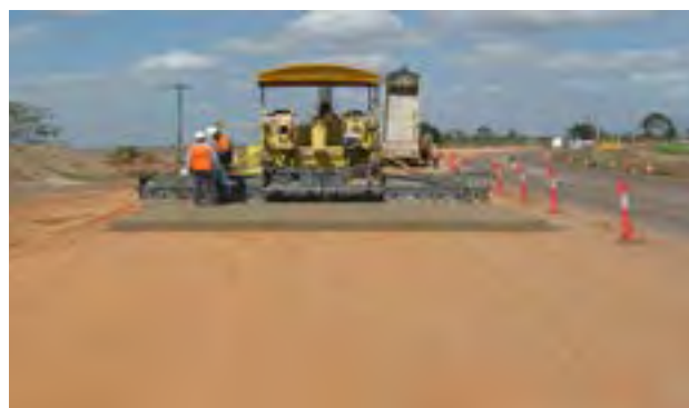
Construction of the Bruce Highway upgrade between Sandy Corner and Collinsons Lagoon is part of the jointly funded Federal and Queensland Government Nation Building Program.
