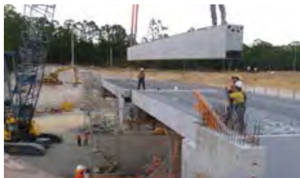
The new overpass forms part of a new 13.5km, four-lane divided highway under construction from south of Cooroy to Federal (near Sankeys Road).
