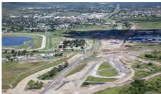
Part of the Nation Building Program, the upgrade will improve safety, capacity, freight efficiency and flood immunity on the Bruce Highway at the southern approach to Townsville.
