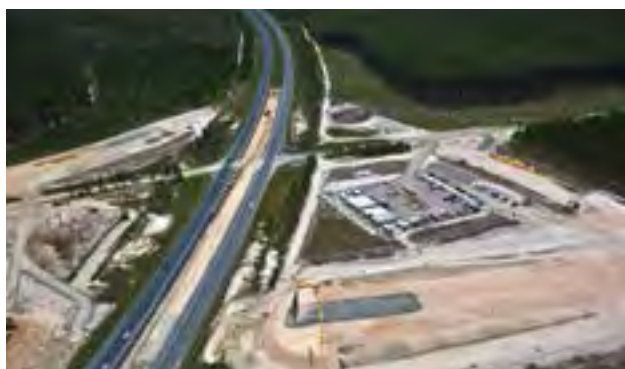
The new interchange will improve safety and efficiency for local and highway traffic, and enhance connectivity between local communities and visitors to the region.
