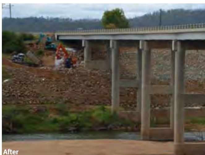
Repairing damage sustained to the embankment of the bridge following flooding in early 2013.
