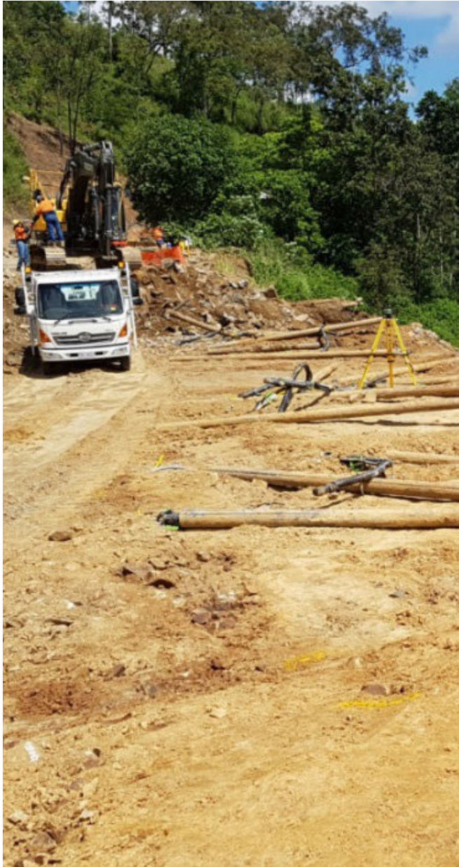
Sarina Range excavation and placement of soil nails at the main slip site.
