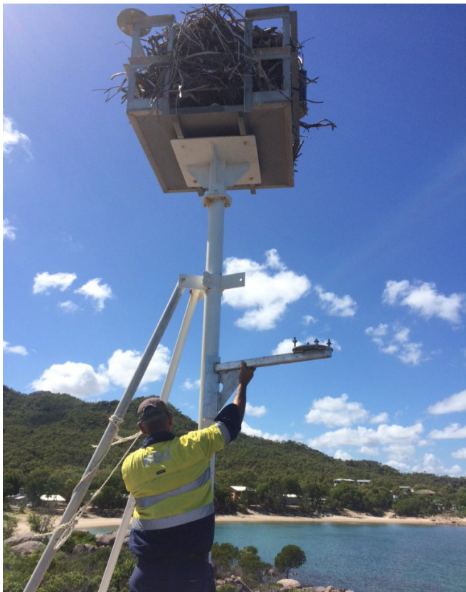
Marine officer installing new navigational light post to protect nesting sea birds.
