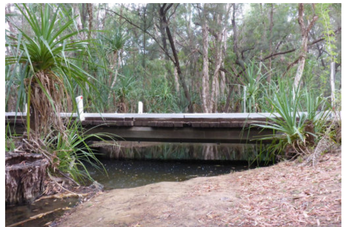
Beames Brook (Julia Creek – Burketown Road) original 1950s single lane timber bridge.
