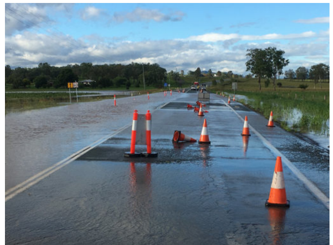
The first layer of foamed bitumen applied to the Warrill View section of the Cunningham Highway prior to the site being inundated by rainfall during Ex-TC Debbie.
