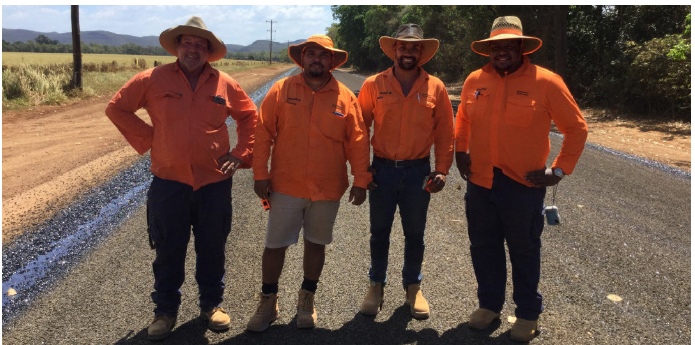
Staff working on the Endeavour Valley Road, Cape York Peninsula, connecting the indigenous community of Hope Vale to Cooktown and beyond.
