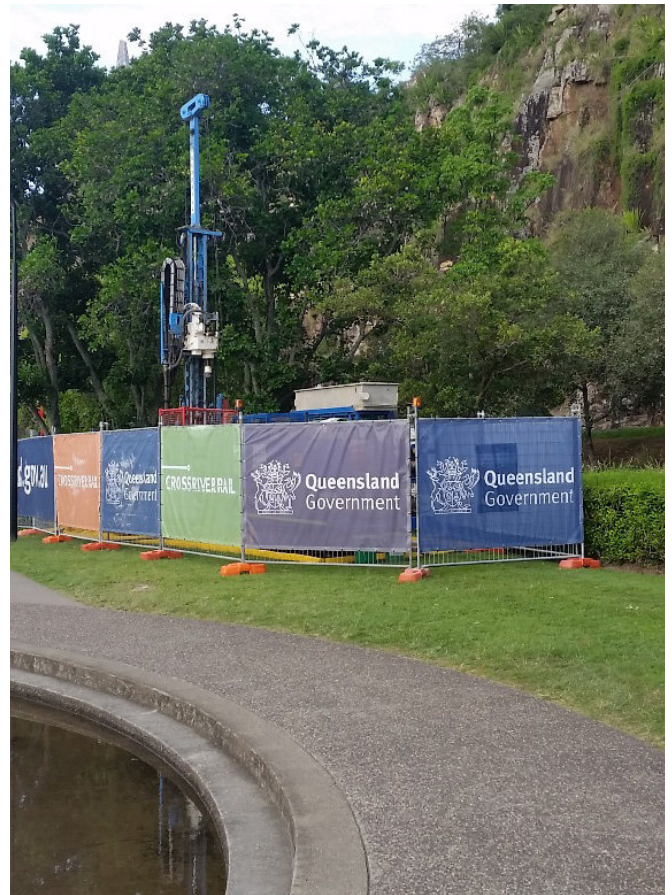
Drilling at the base of Kangaroo Point cliffs—the future tunnel will pass under this area.
