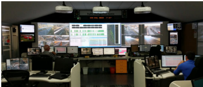
The statewide Operations Interactive Map is a powerful new tool for Traffic Management Centre operators.
