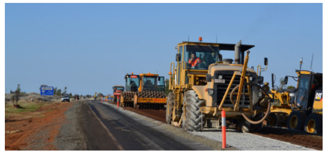
Pavement rehabilitation and overlay, extension of road width and sealing on the Landsborough Highway between Augathella and Tambo.
